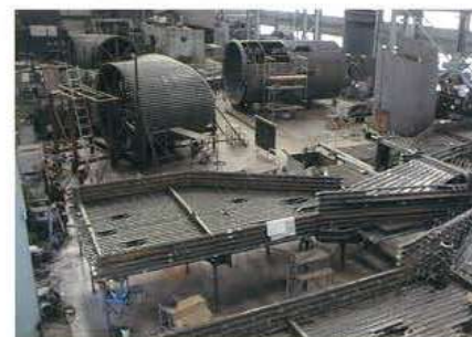
廃熱ボイラー Heat recovery boiler for a gasification & melting furnace for municipal waste incineration
