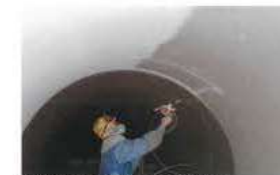
煙道ダクトの現地防食溶射施工 On site wire spraying of the flue
