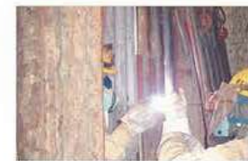
ボイラー水冷壁部分更新 Partial replacement work for the water-cooled wall
